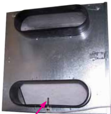
Temperature sensor mounted in fresh air inlet
